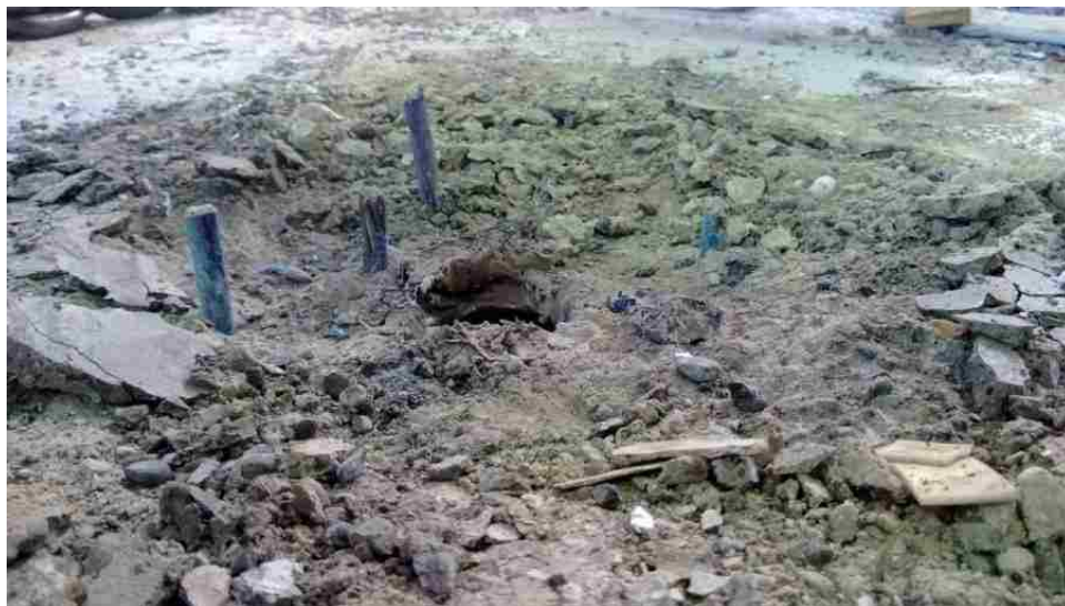
Figure C.7 Top of footing after testing.
