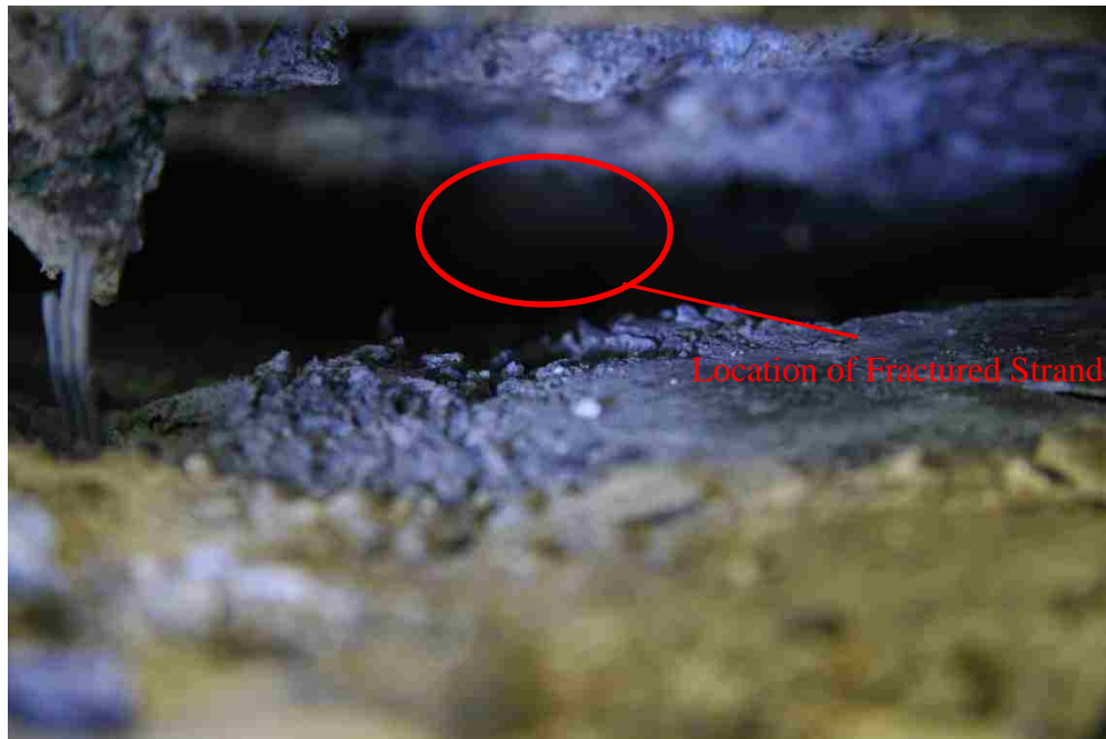
Figure 4.12 Northwest view of PreT-SF-ROCK-HyFRC showing location of missing strand (fractured).
