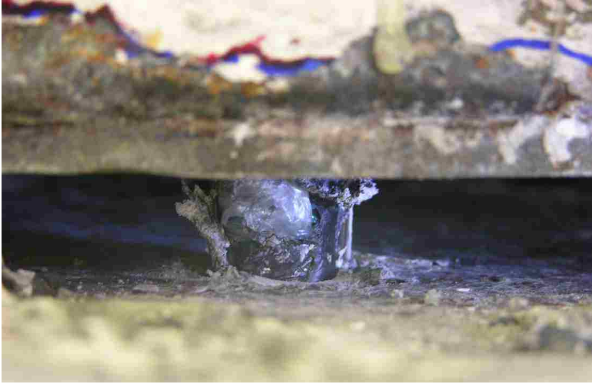
Figure C.11 Exposure of rebar.
