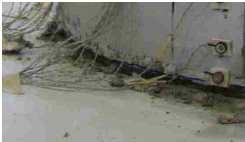
Figure 4.7 South view of PreT-SF-ROCK-HyFRC showing the fillet spalling of the footing induced by the rocking action of the steel shoe.
