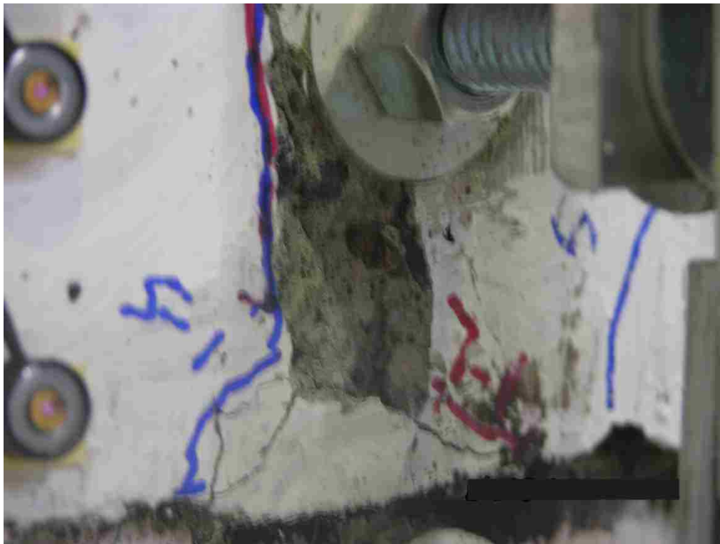
Figure 4.5 South view of PreT-SF-ROCK after cycle 8-4 showing spalling damage above the steel shoe.
