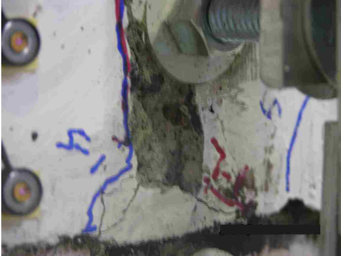
Figure C.9 Cosmetic spalling at top of shoe.
