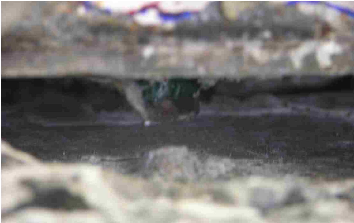
Figure C.12 Fracture of rebar.
