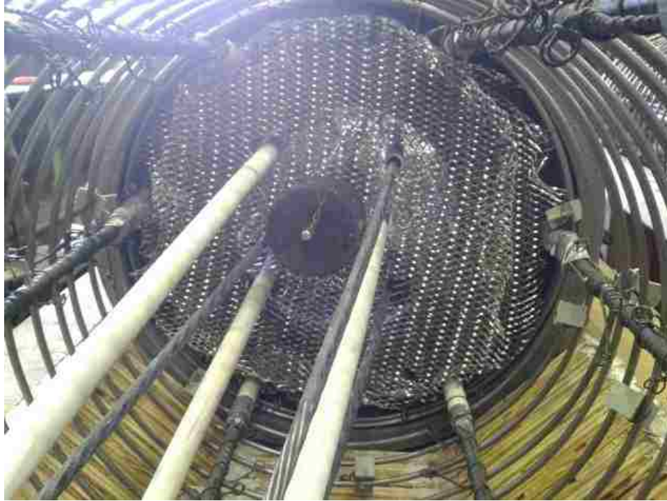
Figure D.2 Dividing mesh used to separate the HyFRC and conventional concrete pours (Image before casting).
