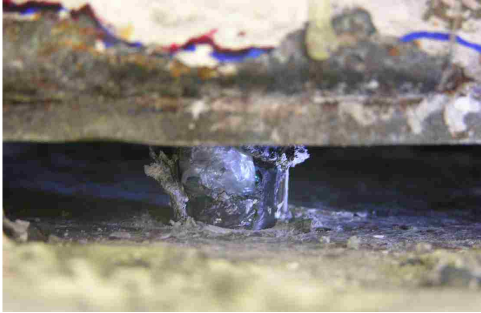
Figure 4.9 Exposed north bar of PreT-SF-ROCK.
